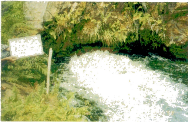
Main Leak Outlet after Significant Reduction of GWL (Leakage Amount 1.77m 3 /s on 13. 09. 98)
