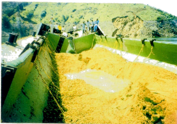
Just before Completion of dropping of Blanket Materials, after about 2 minutes from Opening
