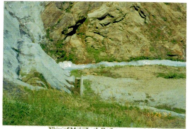
View of Main Leak Outlet
