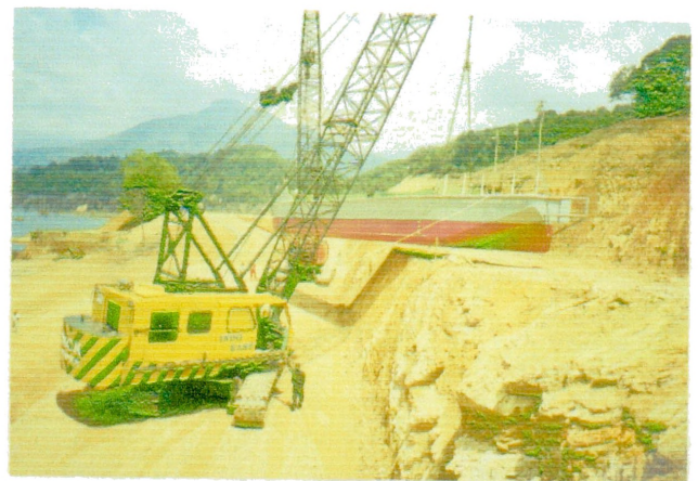
Transportation of an Half Hull of Barge Using 2 nos-80 ton Truck Cranes from El.462 m to El.447 m through Access Road
