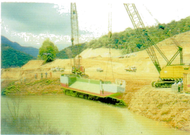
Launching of an Half Hull of Barge Using 2 nos-80 ton Truck Cranes (14-17.03.98)
