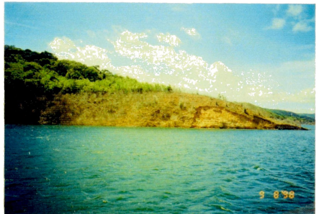
Major Ingress Area Identified at Block X (Right Abutment)
