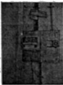
Figure: 1. control meter
