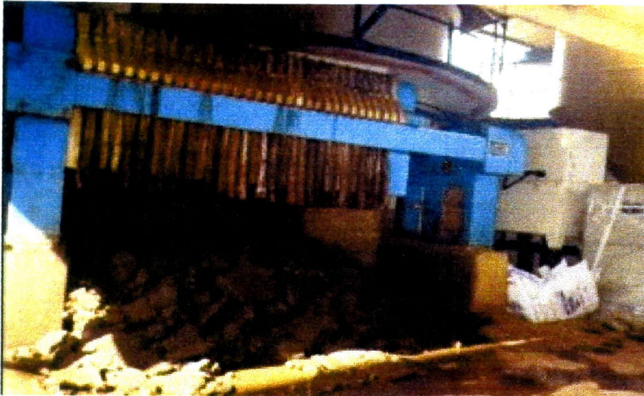
Figure 4.5 Filter Press Machine of Stretchline Wastewater Treatment Plant.
