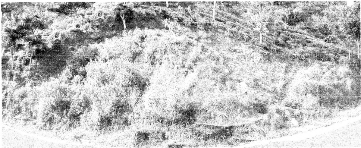
Plate 4.4 :- Minor land slide occurred in a poorly managed tea plantation.
